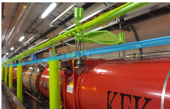
Figure 4: Photo of the low-beta magnets before the physic detector. The alignment systems are highlighted: Hydrostatic Levelling System with water network, support pillars and sensors (light green) and the Wire Positioning System with sensors, stretched wire, wire protection system (light blue).
